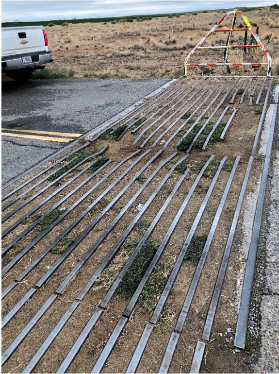
Cattle Guard Silt & Damaged Grates (Before) (After)
