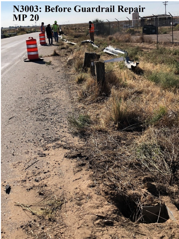
Route N3003 – Guard Rail Damage (Before)
