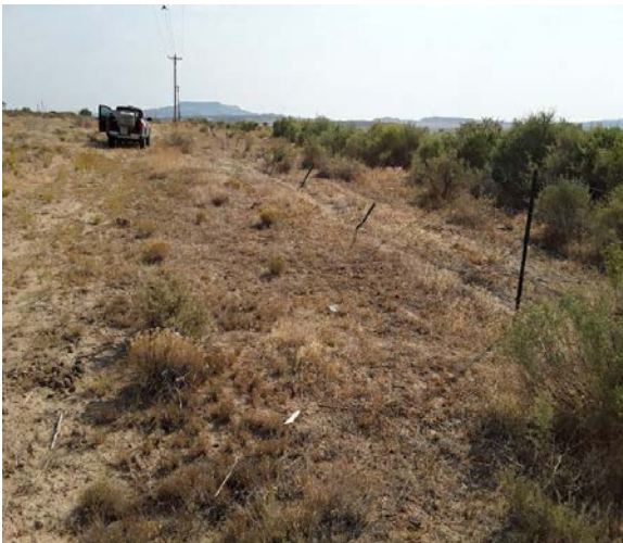
Route N4 – Fence Repair (Before)
